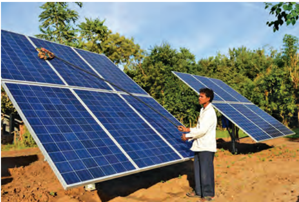
Solar panels - Non-Conventional Energy Source
